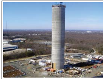
Brandon Shores Power Plant, MD
