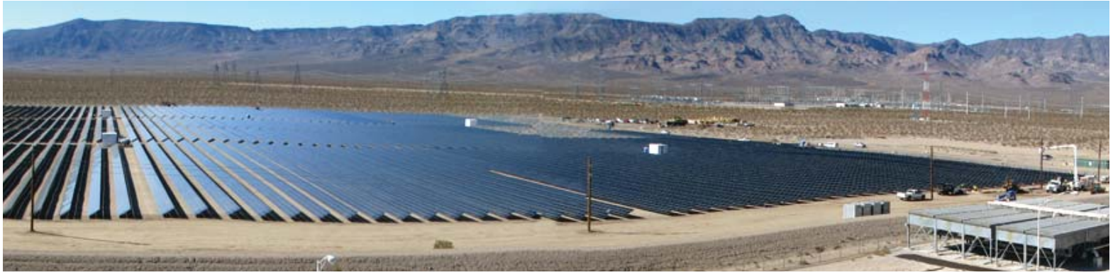
Solar Power Plant Expansion, NV
